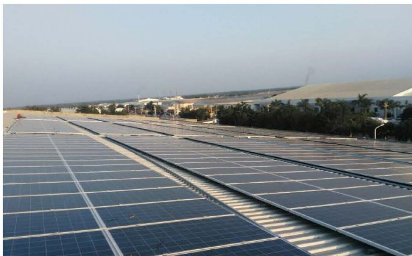
One of SWELECT Energy Systems' Projects
